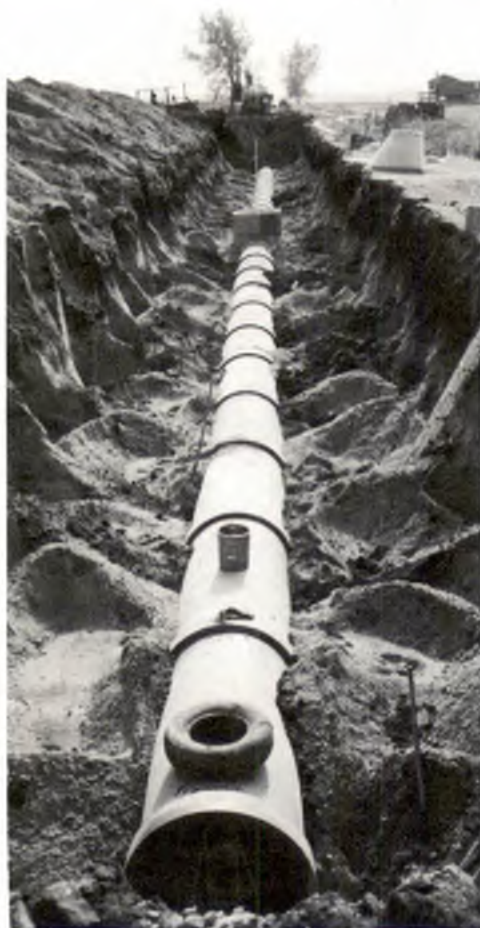
Concrete line coming from the southeast part of town. More than eight miles of 30-inch pipe comes from town to the wastewater plant. The size of the line is large enough for three times the flow Brookings customarily experiences.
