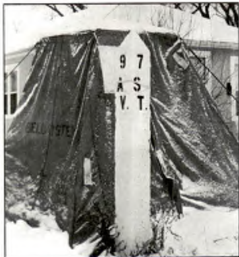
A canvas tent offered a measure of protection from the elements when cable repairs were made in the winter. This was a familiar sight in the 1940s and '50s.
