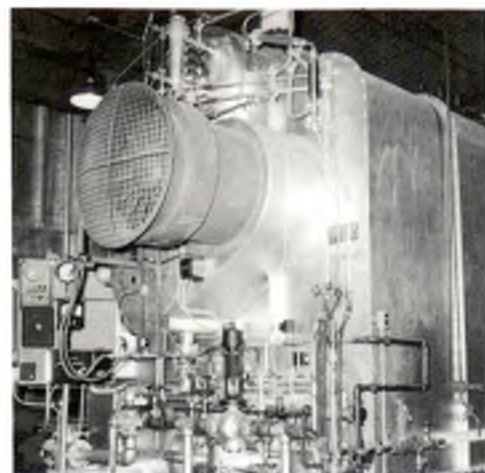
A package boiler used at the power plant. It was operated either with fuel oil or natural gas. The big boiler in the background could use coal, natural gas or fuel oil.
