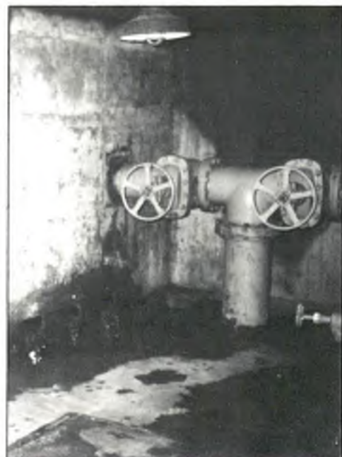
Underdrain of trickling filters at the end of their life span. Because of sulfur dioxide buildup, concrete was pitted, pipes were rusty.
