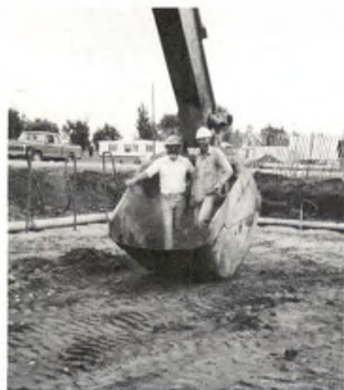
Rollie Harrington, supervisor of water/wastewater during the construction of the new plant, and Bill McMacken, J.T. Banners, standing in the bucket of a big backhoe at the site of the new plant.
