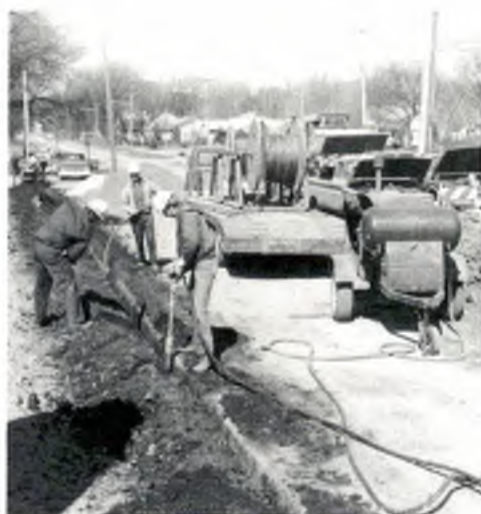
Dennis Merchant places cable in the ground while Tom Honkomp and Jerald Hetlet cover the trench. Cable was to service homes along a stretch of Sixth Street.
