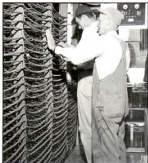
Wires secured to wooden beams caused many a headache for repairmen before the telephone department converted to dial. Knute Knudsen and Earl Bain check the system in the 1940s.
