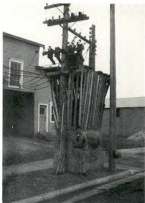
After a child squeezed into the protective structure enclosing a transformer, the city decided it should mount transformers on platforms well above the ground. This photo shows an early transformer near Sexauer elevator.
