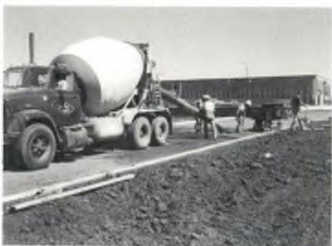
The last stages of construction of the wastewater plant. Sodding was completed and some grass had been planted next to the building. A crew is pouring the concrete street in front of the building.
