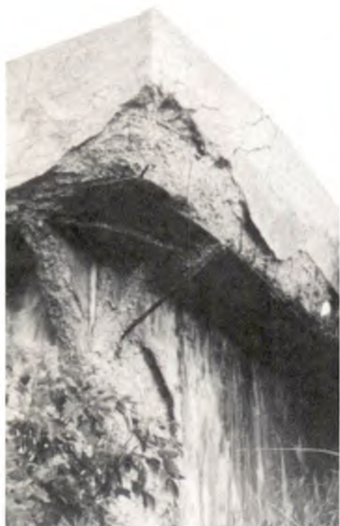
Northwest corner of settling basin, ready to collapse in early 1950s.
