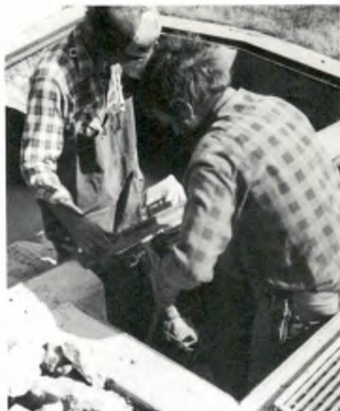
Workers in 1980 cutting in the new line so that wastewater would flow to the new plant rather than the old.
