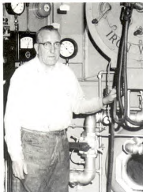
Norm Amundson in the 1950s in front of Erie City boiler controls. Amundson's responsibility was power plant maintenance.
