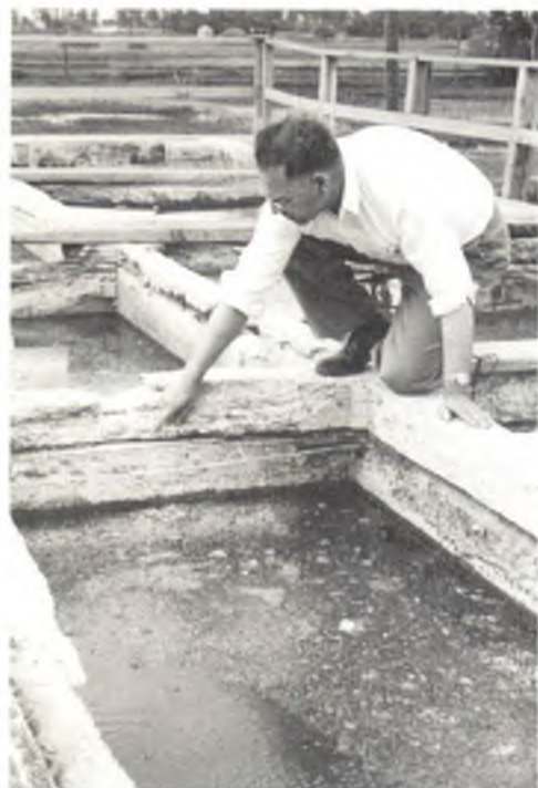
Deteriorating condition of settling basin tanks and flood building compartments shown in 1950 photo.
