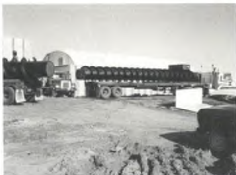
Wastewater flows by gravity to the plant. Once there, it has to be lifted about 18 feet into the plant by screw pumps. Pictured here as they arrived for installation at the plant are two of three pumps. Two pumps are ready for use at any time, the third is backup for maintenance or repair. Each auger can pump 5.25 million gallons a day.
