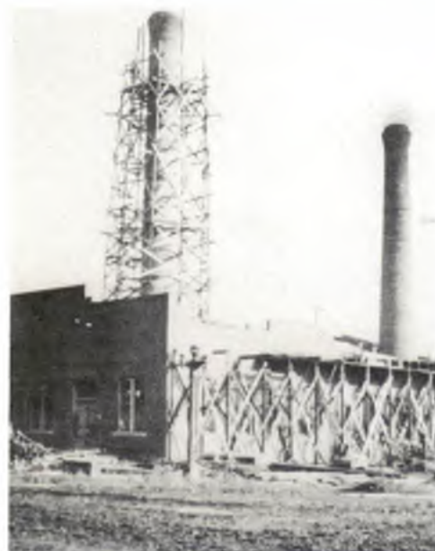
Power plant expansion started in the mid 1920s. Citizens had rejected a proposal to build a new plant but approved a $60,000 bond issue to improve the building and erect a new smokestack.
