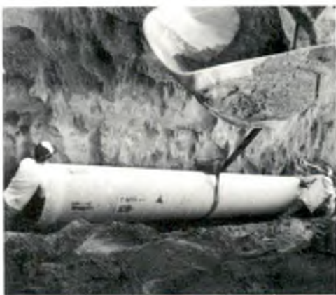
Installation of one of the fiberglass composite pipes for the main line coming to the new plant from the southwest side of Brookings. A large backhoe lifts and sets pipe in a cut. Construction was started in spring of 1979 and continued through fall of 1980.
