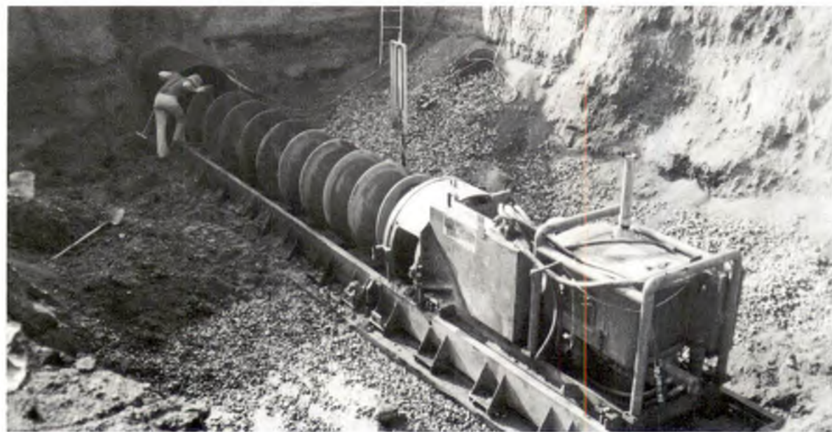
To get across the highways without tearing them up, a hole was dug on either side of the highway. A steel sleeve was inserted and the pipe was run through the sleeve.
